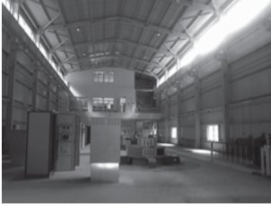
Akdere HEPP 2x3,065 MWm, 2x2,975 MWe 1x1,550 MWm, 1x1,530 MWe
