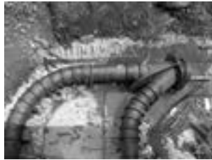
Vizara HEPP Penstock Branches
