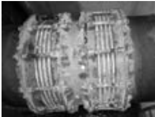
Pařa HEPP Penstock, Flexible Joint
